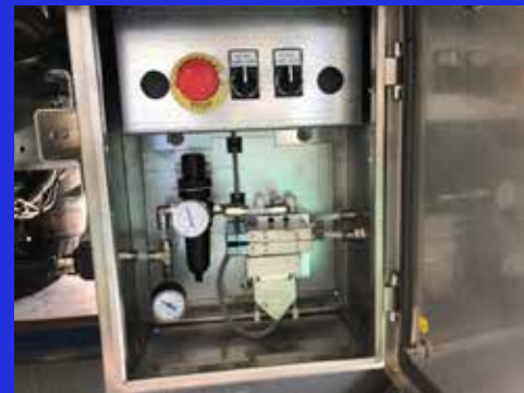
1. ELECTRIC PNEUMATIC CONTROL PANEL
